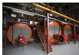
Boilers & Process Heat
